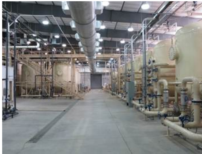
Image: Ur-Energy’s Culver-Douglas Processing Plant at Lost Creek
