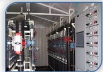
Interior of Header House
