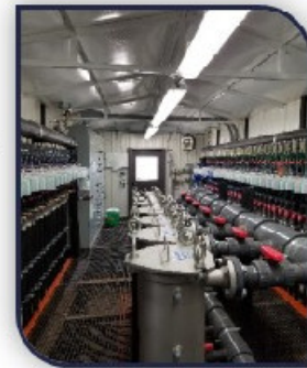
Inside Lost Creek MU2 Header House
