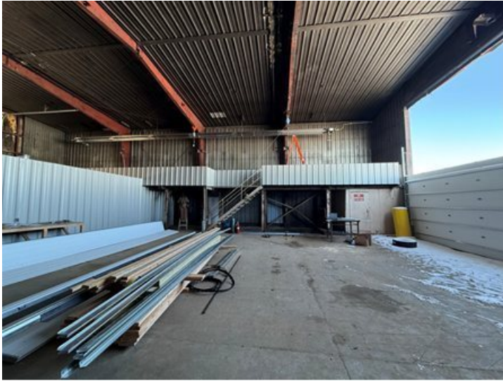
Interior of the conventional mine “wash bay” that is being updated for use as a drilling and logging building. Total square footage is 4,400.
